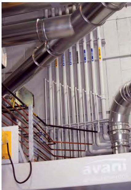
Fig. 4 — The gas manifold system, energy-efficient exhaust snorkels, and safety plugs are part of the 50-year-old welding shop's remodel. (Photo courtesy of Wendy Wright, PCC.)
